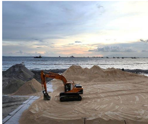
A bulldozer is seen working on the "white sand"—actually crushed dolomite rocks—poured along the shoreline of Manila Bay on September 6, 2020. The STAR/Miguel de Guzman
