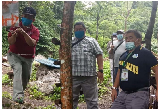
Illegal structures and fences/enclosures erected by a fraternity inside the upper Marikina Watershed and Masungi Wildlife Sanctuary in KM 45 Marcos Highway, Pinugay, Baras, Rizal, were demolished on July 30. The team was led by Executive Director Nilo Tamoria (left) of the DENR's Environmental Protection and Enforcement Task Force and Undesecretary Jim O. Sampulna (center).
